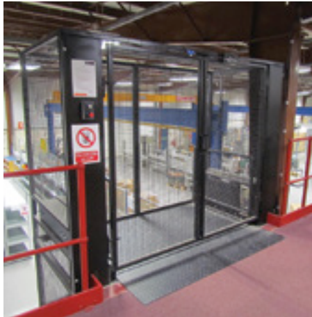
Interlocked gate at upper level
